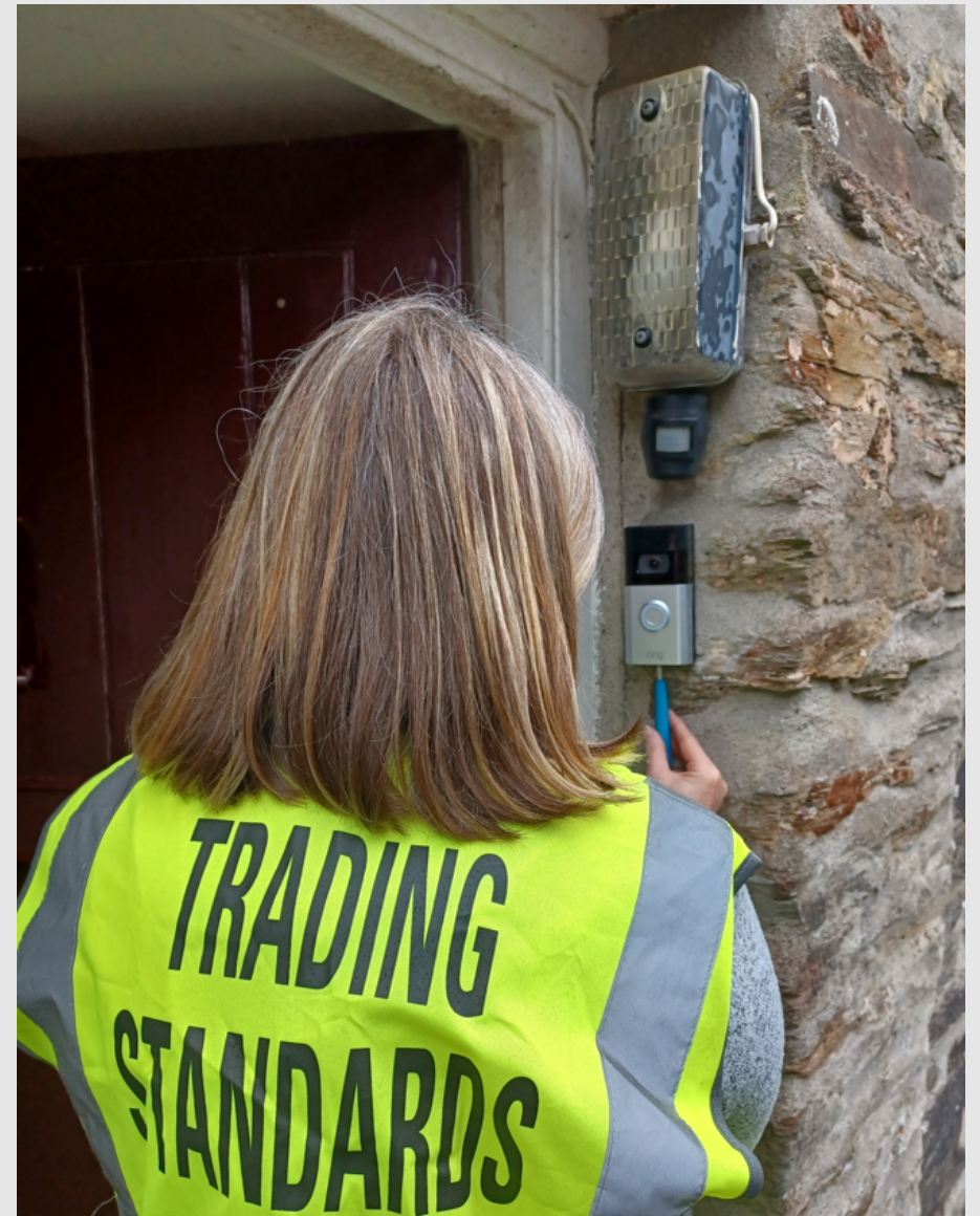
We have installed video doorbells at the homes of repeat doorstep crime victims using money from Proceeds of Crime
